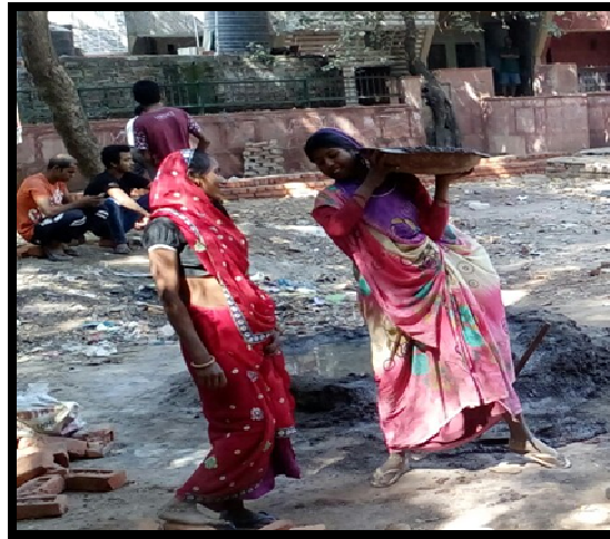
Figure 1: Cement Porters Working Without Protective Clothing
